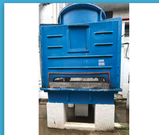
Cooling Tower In Moulding
